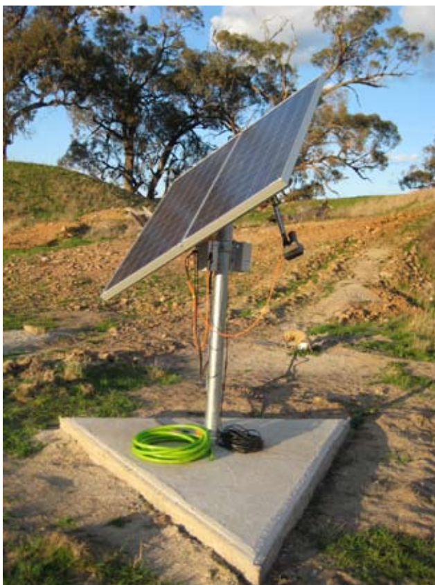
Rotating solar panels
